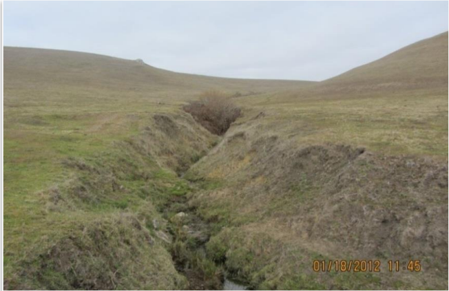
Pre-construction Photo 01/2012 Upstream view before riparian fence and grade stabilization repairs were installed.
