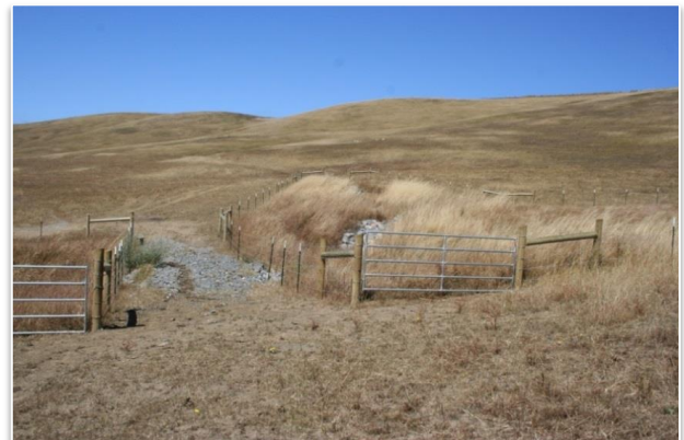
Post-construction Photo 06/2015 Project site after construction showing the riparian fence encompassing the gully headcut and bordering a livestock culvert crossing repair
