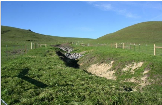
Post-construction Photo 01/2015 Upstream view after construction of the following practices: riparian, fence, grade stabilization repairs and revegetation.
